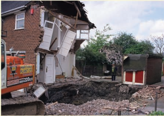
Collapse of old mine shaft forgotten beneath restored site, Walsall.
