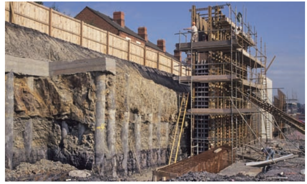
Retaining wall under construction, with frontal toe, rear heel and buried shear key, for new road cut in Midlands; exposed bored piles provided temporary support.
