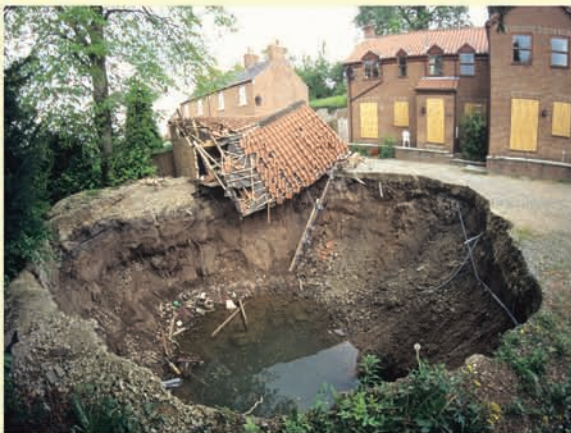
Sinkhole collapse in soil and rock over buried gypsum, Ripon.
