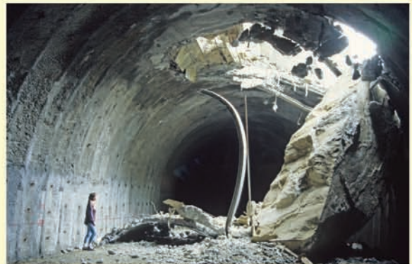
Lined tunnel, too close to hillside, destroyed by landslide, Taiwan.
