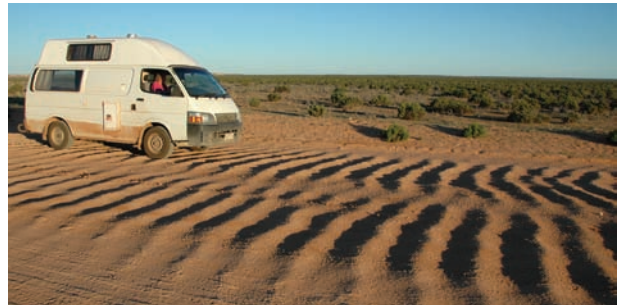
Corrugated road on dune sand in Australia.
