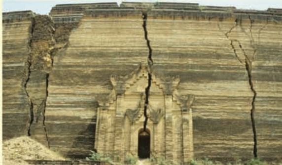
Earthquake damage to temple built on alluvial sand, Burma.
