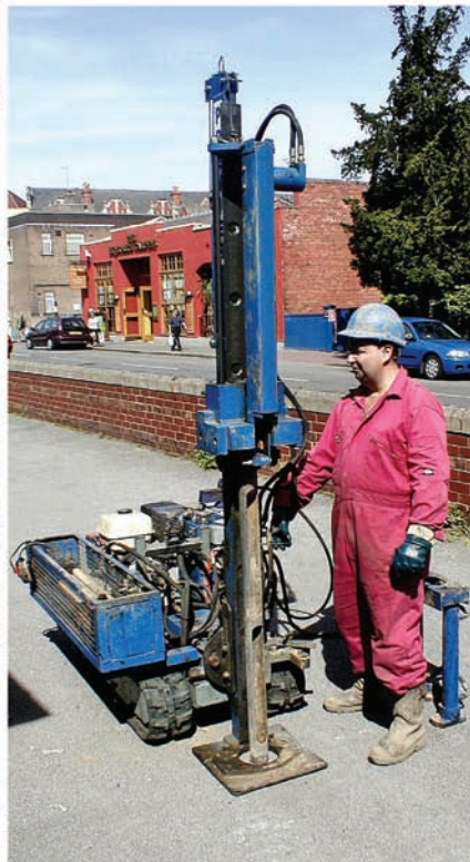
A mobile window sampler unit set up and ready to drill through a compacted gravel surface into the soil profile of a site in England.
