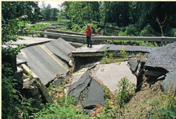
Subsidence sinkhole near deep limestone quarry, Pennsylvania.
