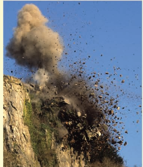
Fly rock from blast of unsafe buttress, Cheddar Gorge.
